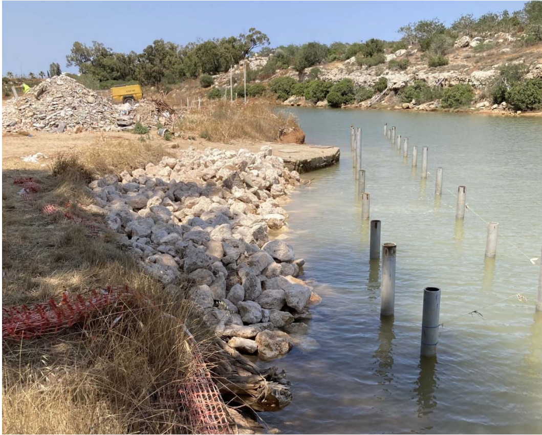
Photo 7. Steel piles have been hammered in place and gabions placed between. Rock armor covers all, matching with the natural environment
