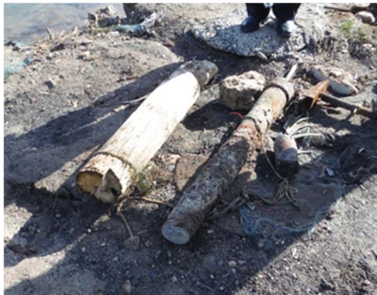
Photo 5. Clear cut of wooden and steel piles using hydraulic disks by divers
