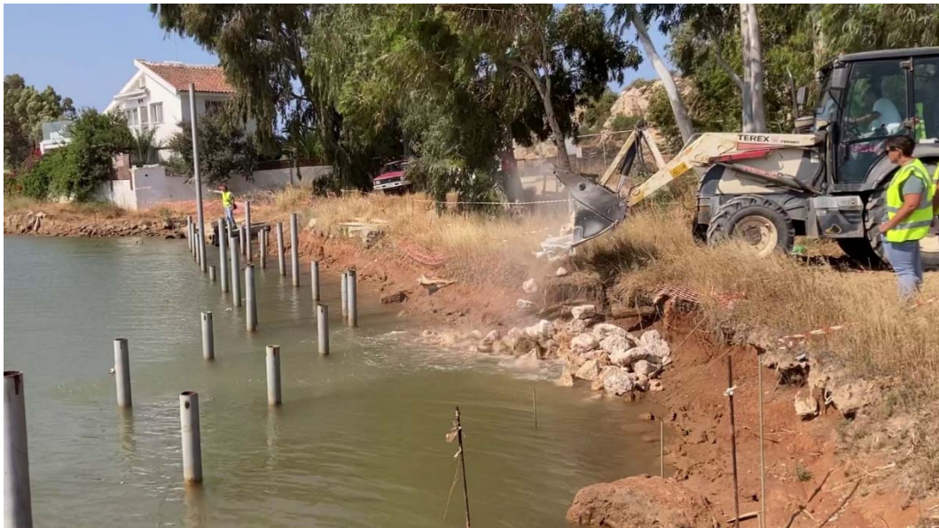
Photo 6. Rock armor is placed on the banks to protect the soft soil, after steel piles' hammering and before any superstructure is installed
