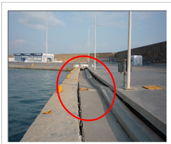
Figure 5: Destruction at the Katakolo port breakwater in 2009
