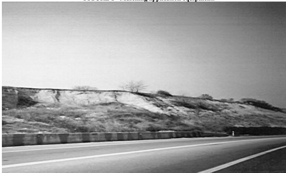
FIGURE 2 - Great soil erosion observed in Area I (left side).
