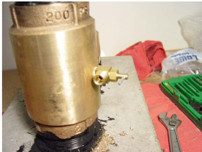
Needle valve installed.
