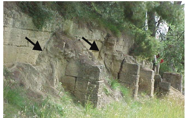
Figure 4. The ancient retaining wall leans due to the occurred earth pressure
