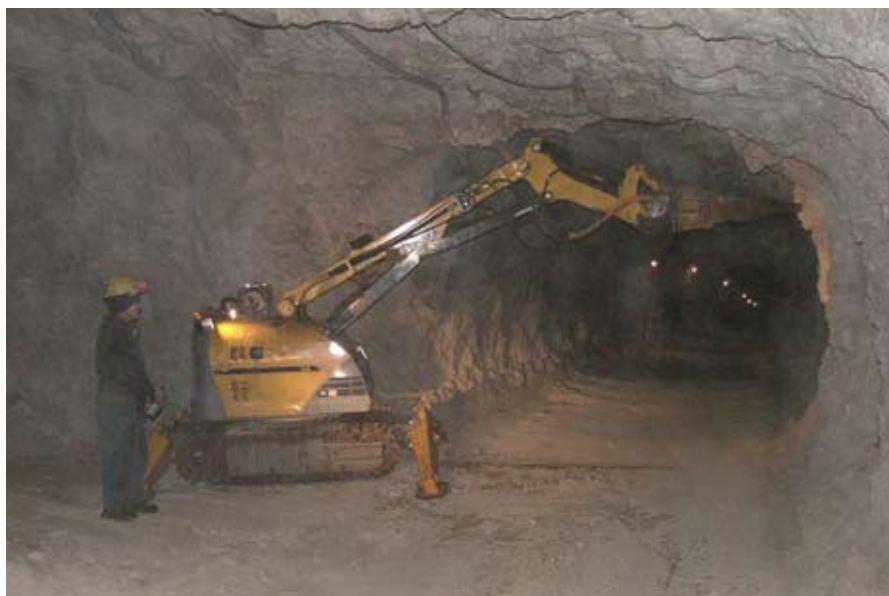
Drilling in Elmin SA's underground bauxite mine near Lamia, on the central east coast of Greece.
